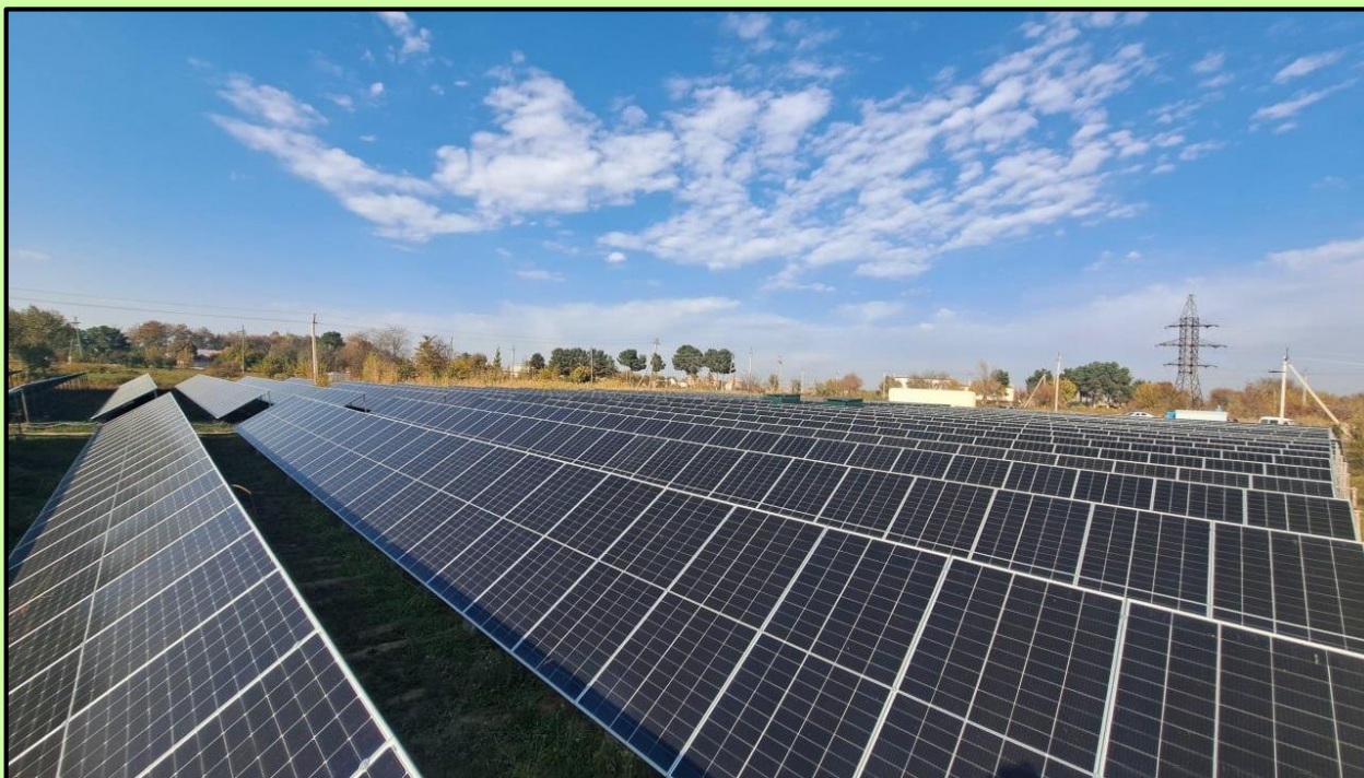
Photo 6: University's solar power station
