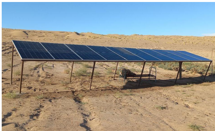
1-rasm. Termiz shahri yaqinidagi 4,5kVt quvvatli FES
